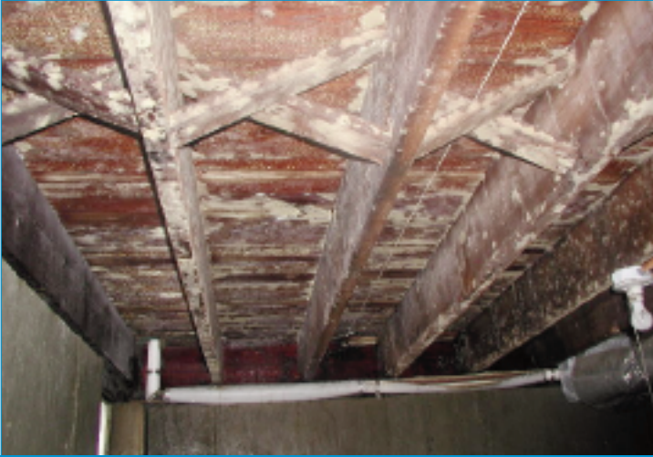
The average mold remediation in a residence costs homeowners between $50-100K.
